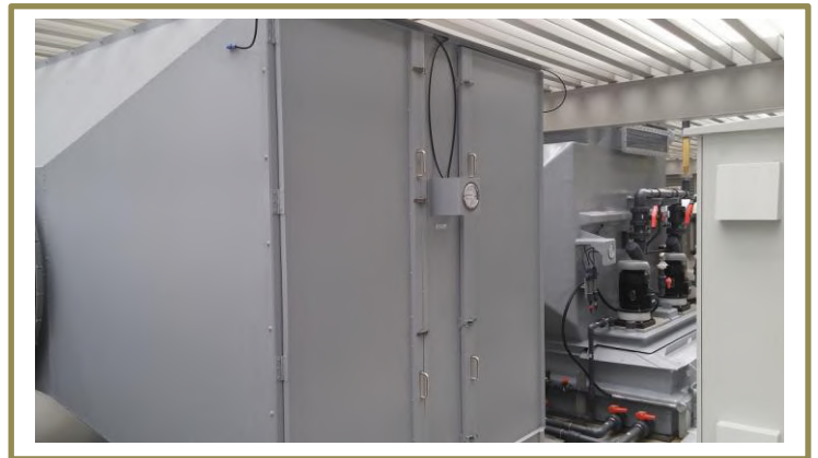
V-Bank ACF with Wet Scrubber Installation for a local university
