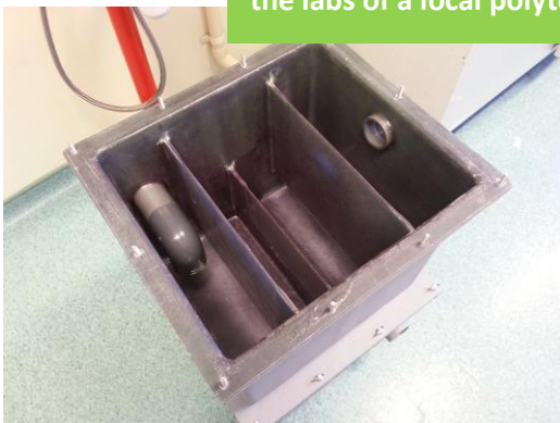
Localised Dilution Tanks for the labs of a local polytechnic
