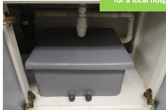
Localised Dilution Tank for a local hospital
