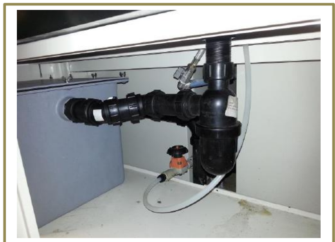
Dilution Tank for laboratories of a local polytechnic
