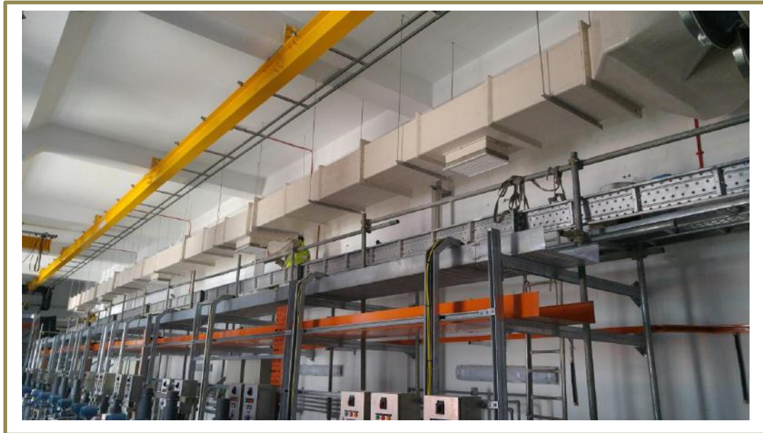
Rectangular ducts for PUB plant
